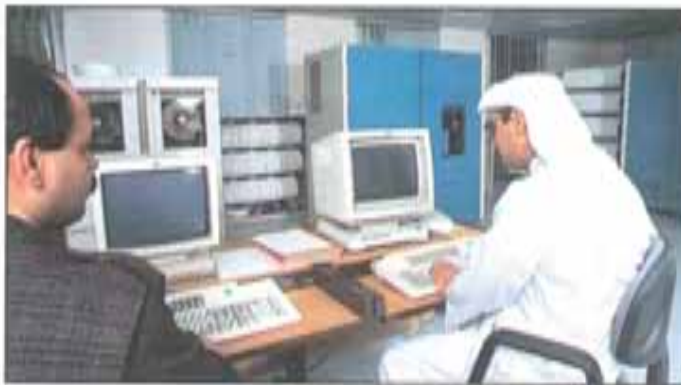
Main frame Computer Room
